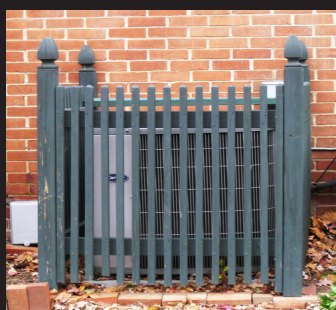
Example of appropriate ground-mounted HVAC screening.
