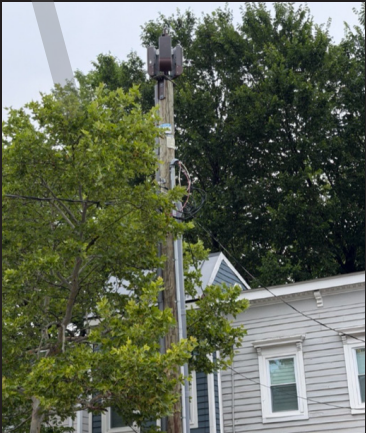
This is an example of a small cell pole installed in the public right-of-way.
