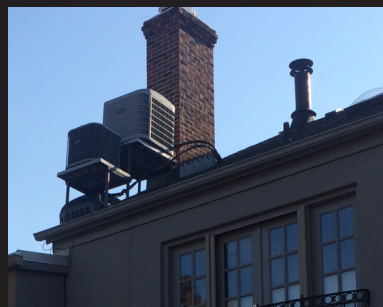
Example of inappropriate unscreened roof-mounted HVAC.
