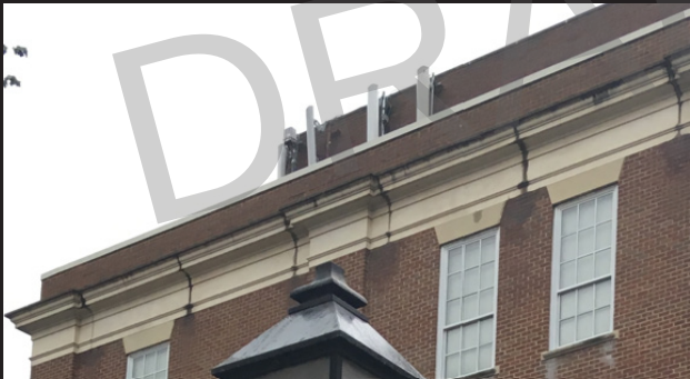
This is an example of penthouse wall mounted small cell antennas.
